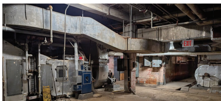
Equipment in BC tunnels./Courtesy of the Open Forum
